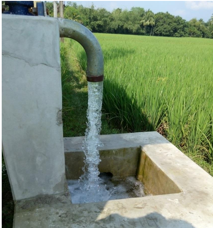
Water output from 5 HP Borewell Pumpset
